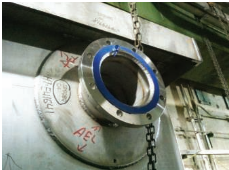
FIGURE 1. This photo shows a reinforced nozzle on a rectangular tank during onsite construction. Note the weep hole located at the bottom of the reinforcement pad
