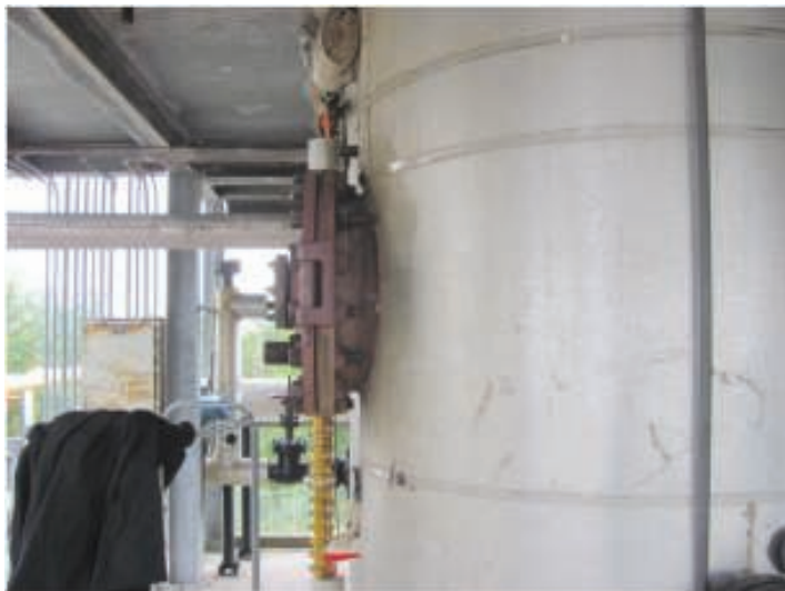
FIGURE 9. Column manholes allow humans and equipment to enter
