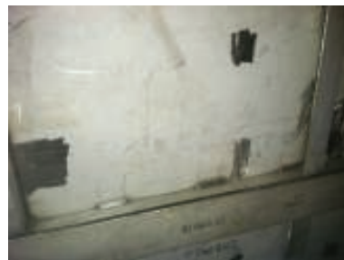
FIGURE 8. On this tank, structural reinforcement is provided by a horizontal 'T' shape that is stitch-welded to the side wall of a rectangular stainless steel tank
