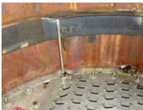
FIGURE 8. New tray rings can be welded to tower walls or they can be supported using posts that are attached to the old rings
